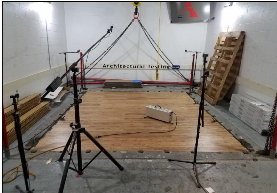
Source Room View of Test Specimen Installation
